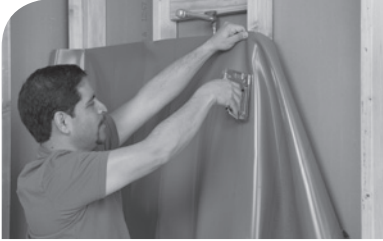
Nail or staple 16 lb roofing felt or 4 mil polyethylene sheathing to studs.
